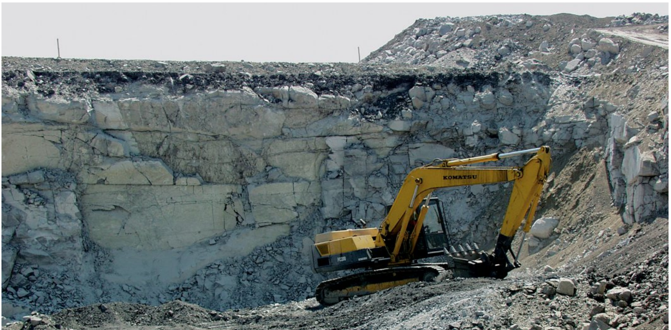
An excavator cleans the top of the MG2 reef. The use of tulip plugs means that the overburden can be removed cleanly without disturbing the underlying chrome ore. To clean the top of the reef, the excavator operator uses the back of the bucket to ensure the chrome ore remains in situ.
